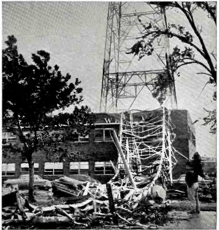
After the storm had done its damage.
